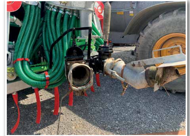
EXISTING FILL POINTS AND SPLASH PLATE RETAINED
